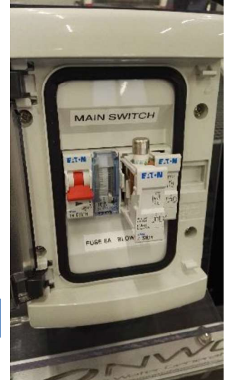
Picture 1. Electric Panel
