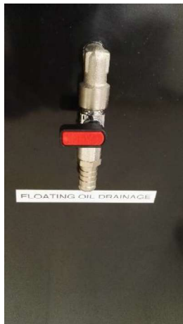
Picture 2. Oil Drain Tap
