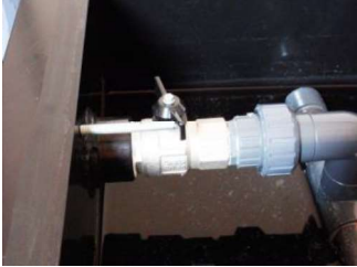
Picture 11 Detail: water input valve (has to remain fixed)
