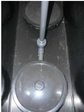
Picture 8 Aeration Tank, detail bottom air diffusion
