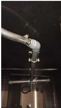
Picture 9 Secondary aeration Tank, detail air piping
